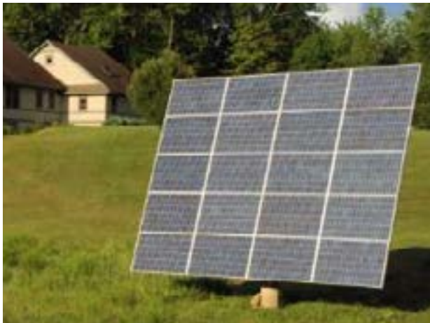
Ground-Mounted Solar Panels in Rear Yard
