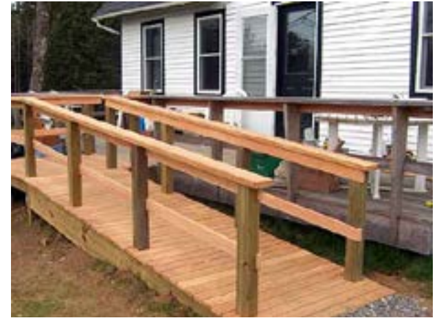
Reversible Handicapped Access on Historic Structure. New Wood Must be Stained or Painted
