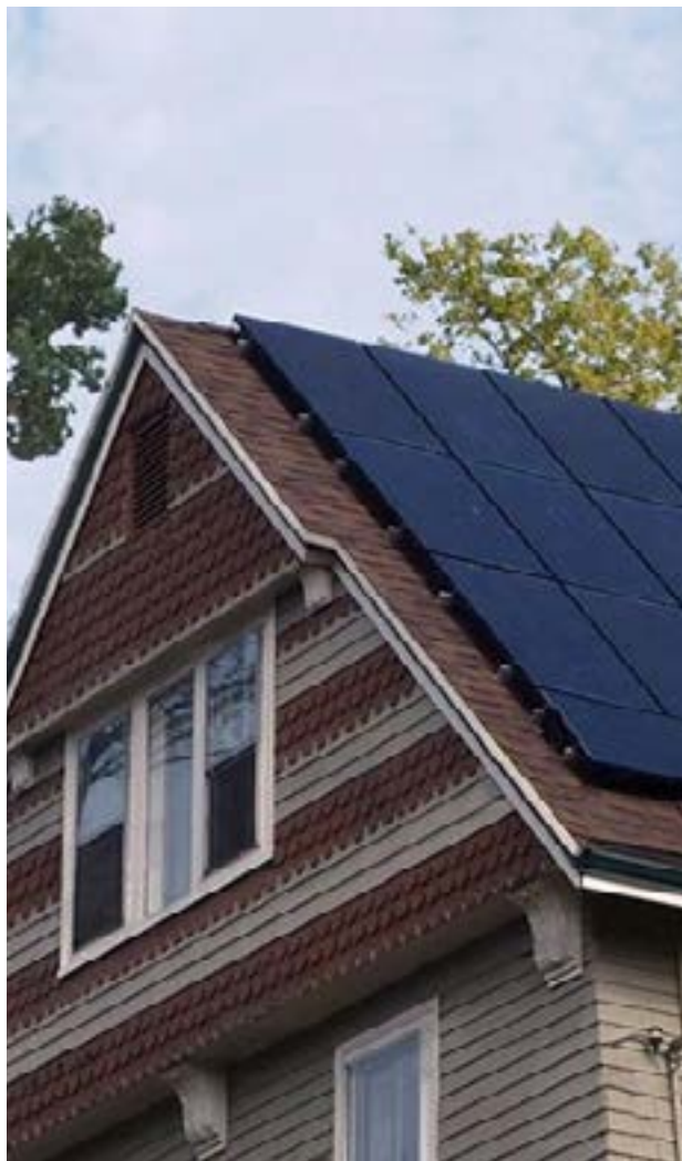
Solar Panels Applied to Rear Roof of Historic Home, where it is less visible from the street
