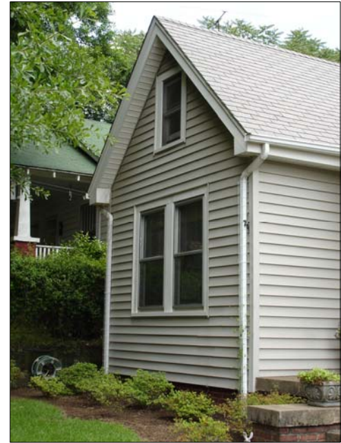
Figure 20: When applied, care should be taken to use synthetic siding material that not only reflects a similar appearance of the original, but also that it does not obscure architectural.
