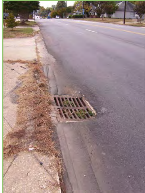
Storm Drainage Grate and drop inlet on North Main Street near 12 th Street.
