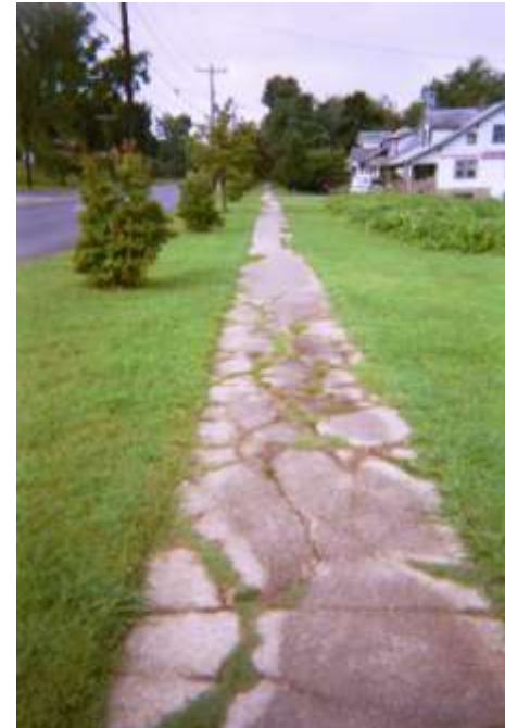
Broken sidewalk in the 1000 block of North Main Street.
