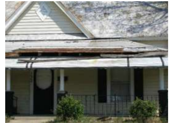
House in deteriorated state.
